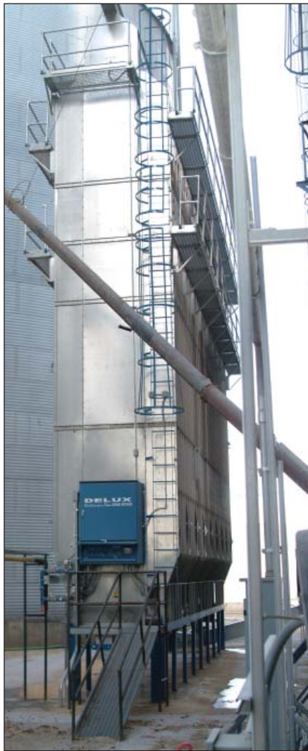
New Delux DPX 16GT328200 dryer installed during the summer of 2014 at United Farmers Mercantile Coop's rail terminal in Red Oak, IA, rated at 3,280 bph at five points of moisture removal. Photos by Jerry Perkins.
